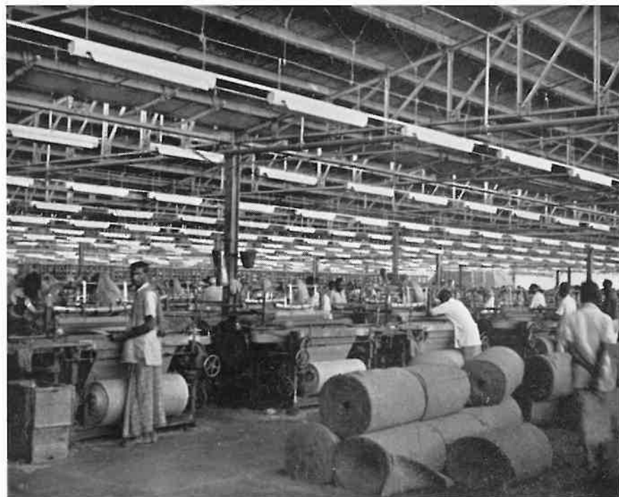
Loom Section of Adamjee No. 1 mill, showing the method by which BTH fittings are suspended by Channel Conduit.
